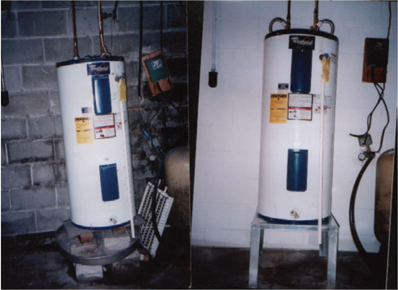
Figure 12-1 Makeshift Attempt to Support a Water Heater (left) vs. an Engineered Solution (right)
